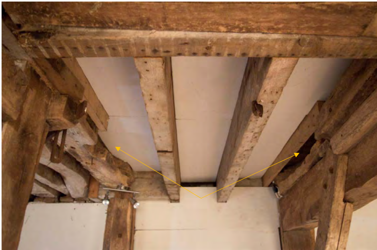
Plate 10 Curved recesses in the girders of the hurst indicating the site of one of the removed pairs of millstones (FMI18-0154)
