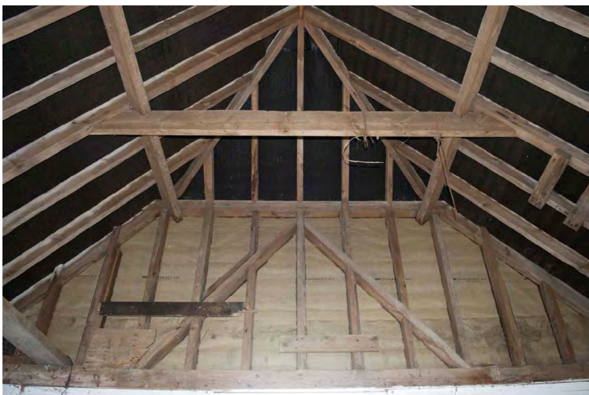
Plate 48 Detail of the half-hipped roof terminal to the south-east of the storage. Note the pair of horizontal timbers nailed to the rafters, to the right-hand side (FMI18-0035)
