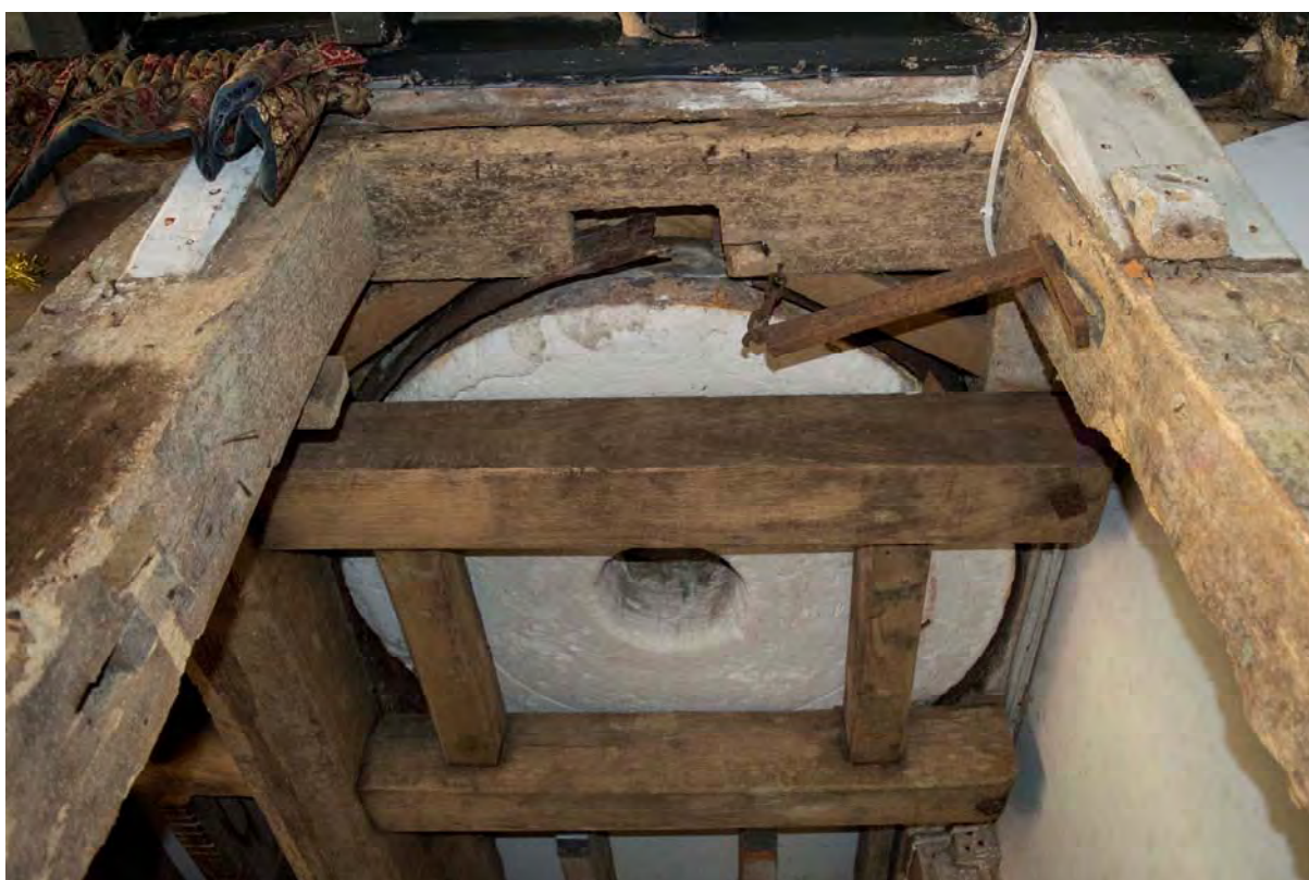
Plate 8 The underside of one of the millstones which remains in situ within the southern bay of the mill. Note the adjoining iron fixture (FMI18-0109)
