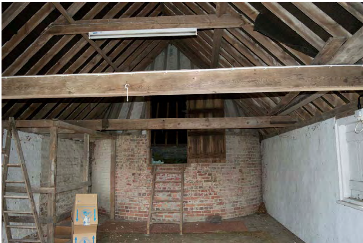
Plate 47 The roundel, viewed from within the storage at first floor level (FMI18-0036)
