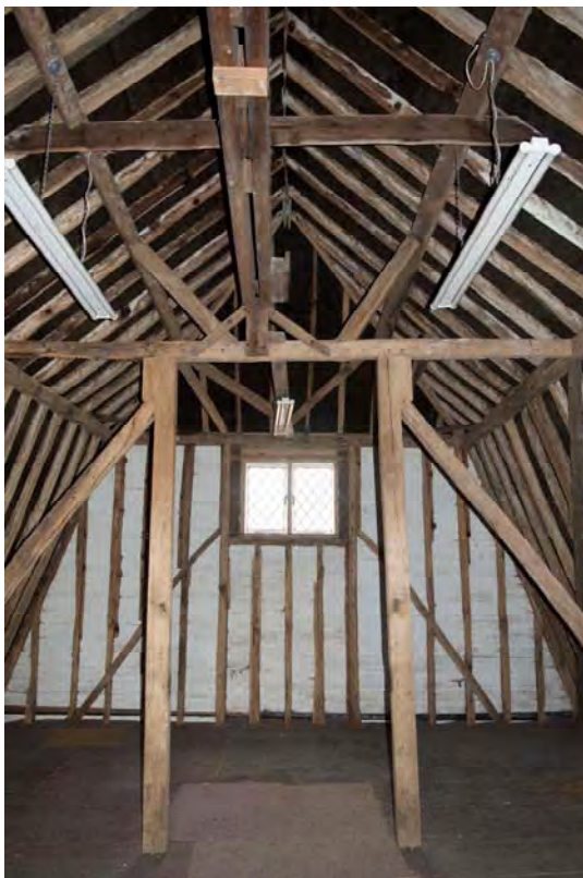
Plate 24 Detail of the truss on the northern side of the central bay, facing north (FMI18-0061)
