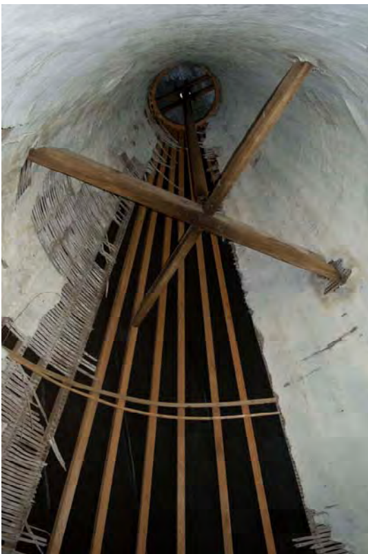
Plate 52 The interior of the conical roof of the roundel, showing the cross-piece and the cylindrical pivot of the cowl (FMI18-0042)
