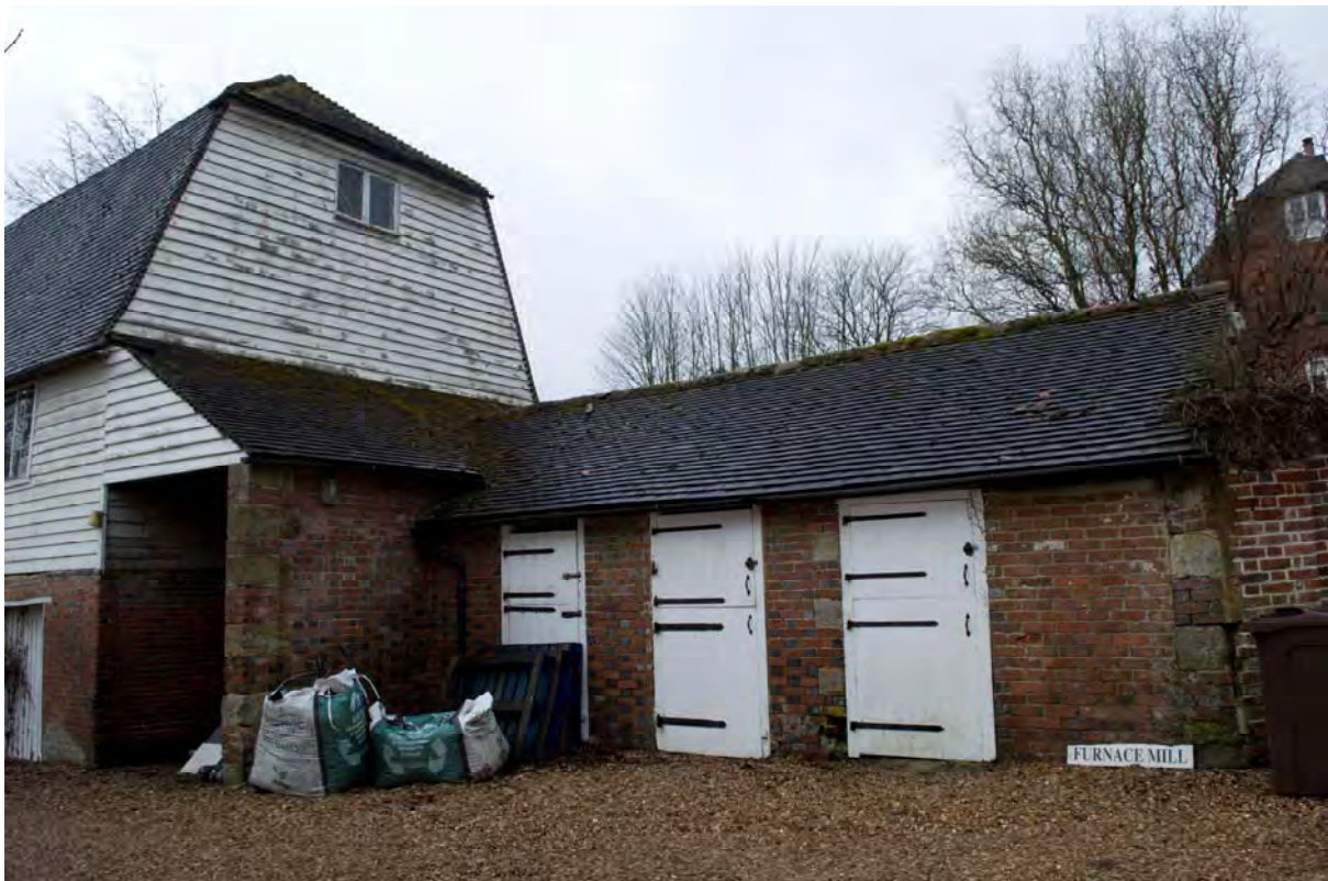
Plate 6 The north elevation of the mill, and the mid-19 th century additions, facing south-west (FMI18-0003)
