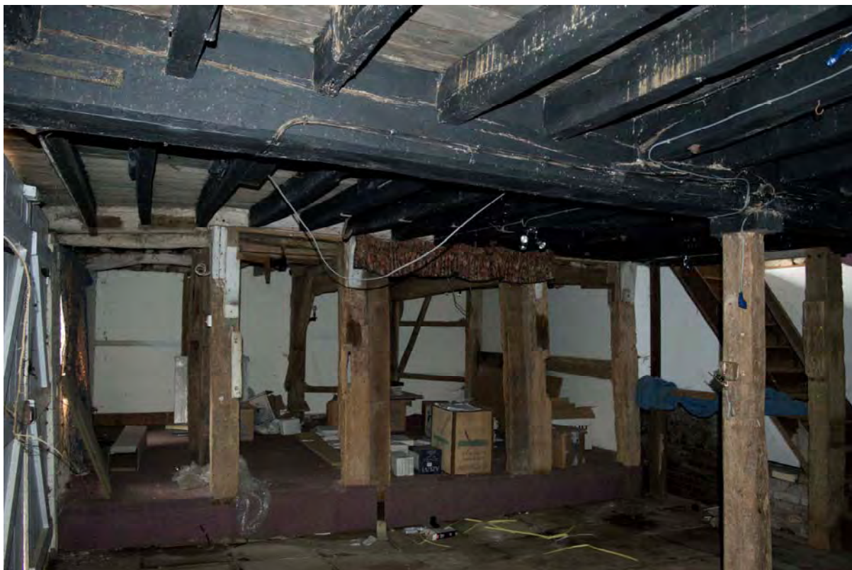
Plate 9 Ground floor of the mill, facing south, showing the hurst which supports the millstones (FMI18-0101)
