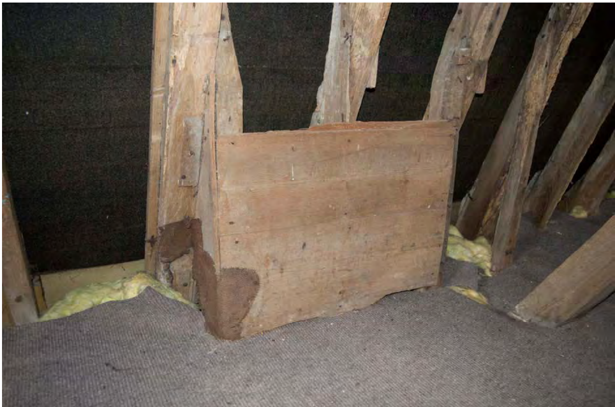
Plate 22 Remnant of horizontal boarding relating to grain bins, on the east side of the central bay at second floor level (FMI18-0066)
