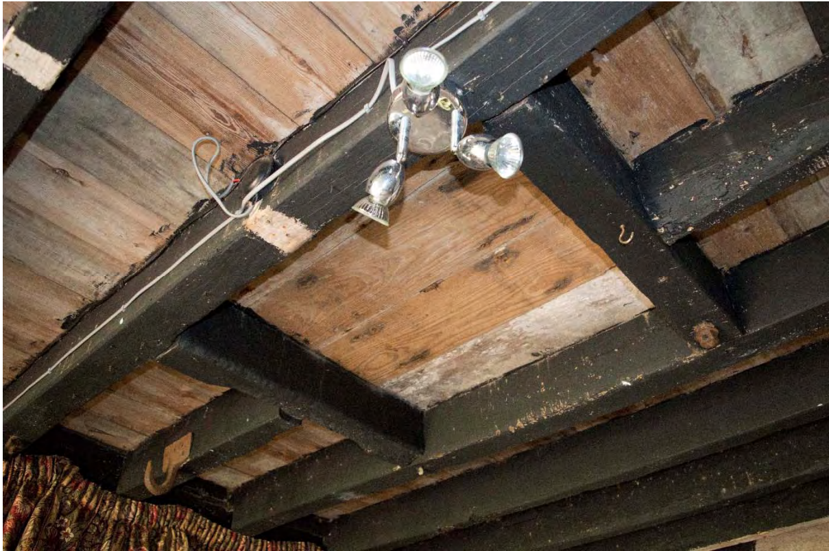
Plate 13 The central trap hatch in the ground floor ceiling, facing south-west (FMI18-0107)
