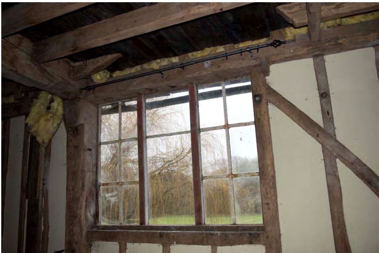
Plate 20 Truncated first floor ceiling joist on the east side of the southern bay (FMI18-0088)
