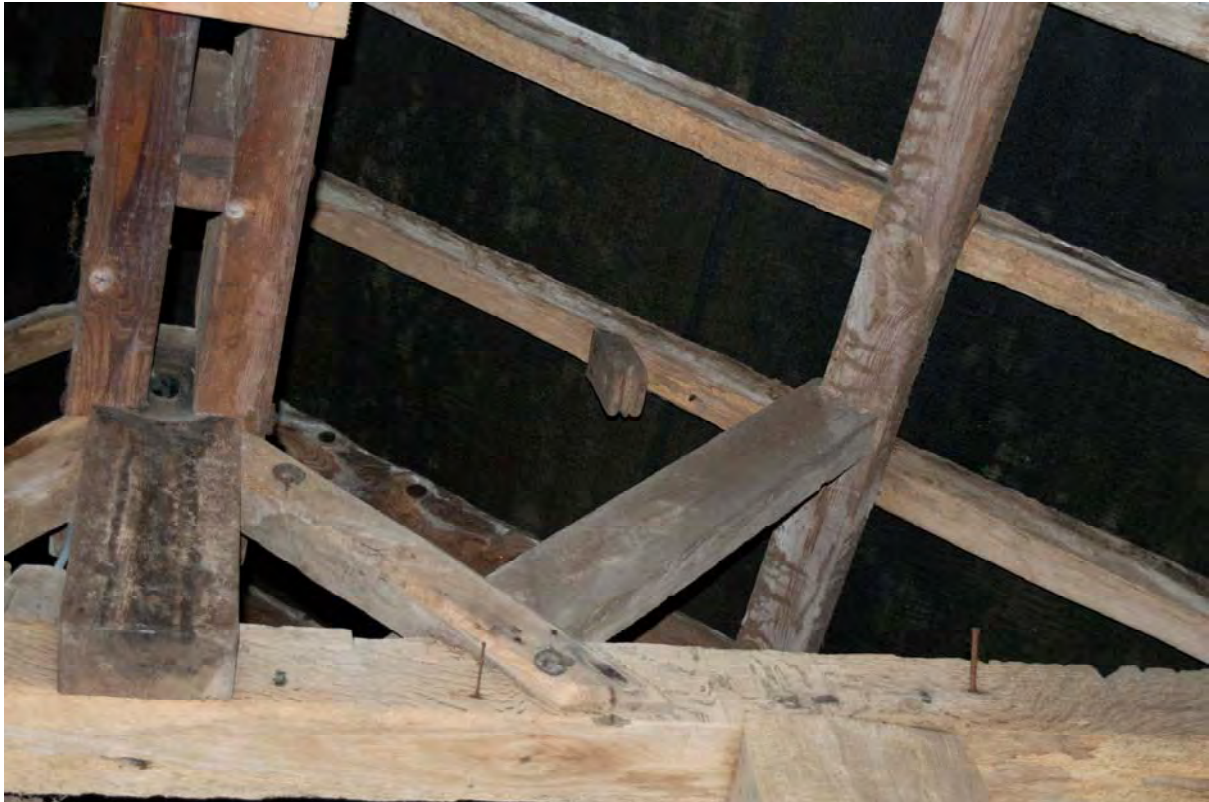
Plate 25 Detail of the arrangement of the support for the sack hoist wheel. Note the timber pulley fixing attached to the rafter (FMI18-0125)
