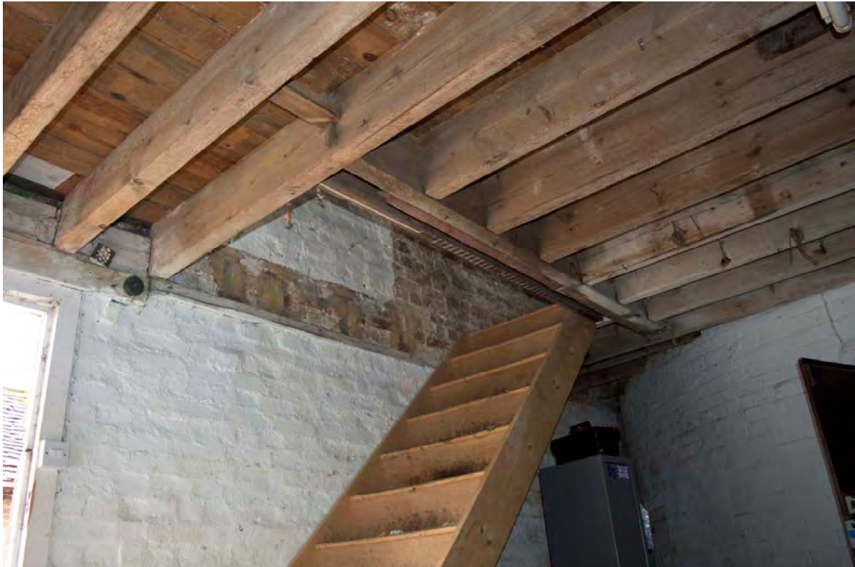
Plate 45 The existing stair to the first floor, which occupies the original stair trap. Redundant joist mortices appear to be for a later alteration. (FMI18-0056)
