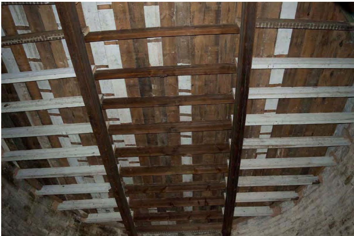
Plate 44 Detail of the construction of the existing first floor structure in the roundel (FMI18-0047)
