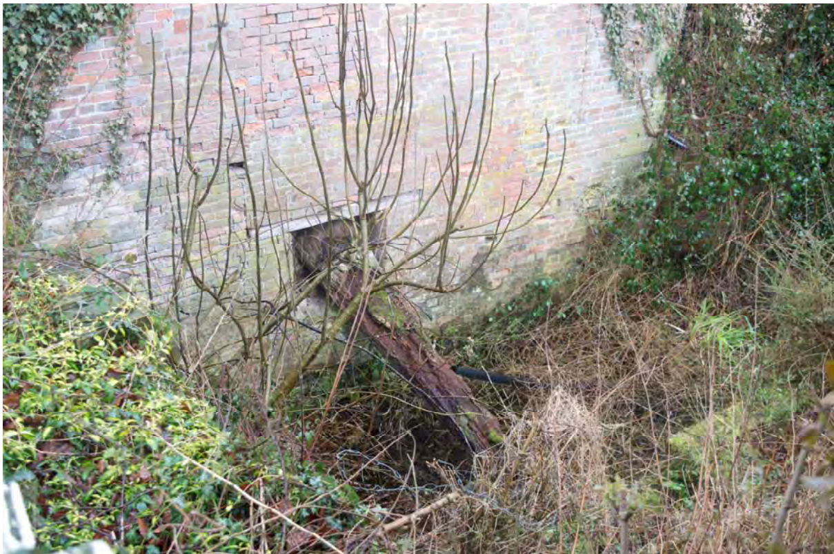
Plate 4 Detail of the timber wheelshaft. Note the coursed stone to the left-hand side (FMI18-0014)
