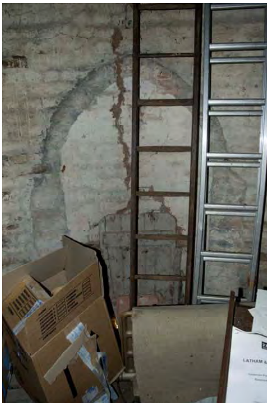
Plate 42 Scars around the probable stoking hole/fuel door to the north-west of the roundel (FMI18-0048)
