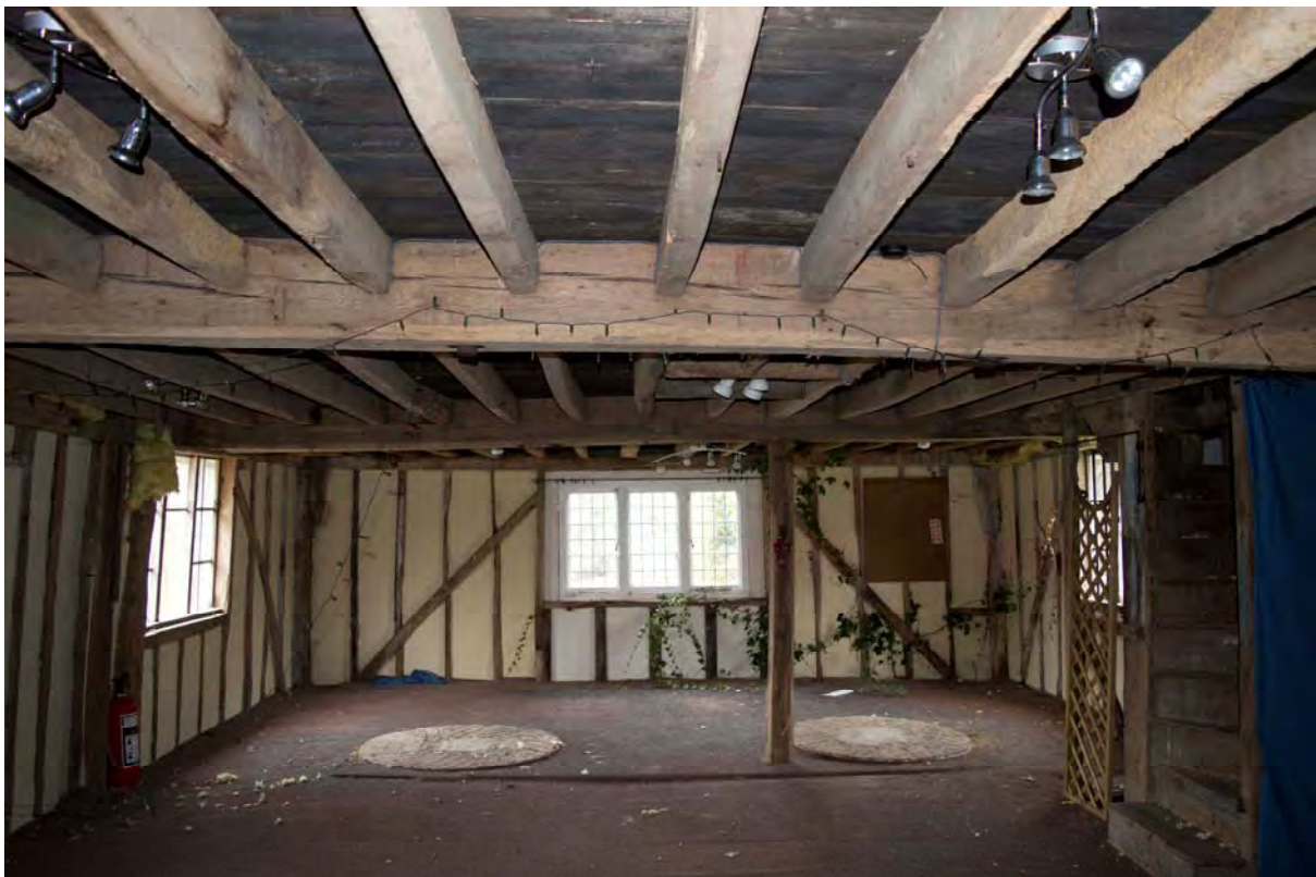
Plate 14 The first floor of the mill, facing south, showing the bedstones which remain in situ (FMI18-0074)
