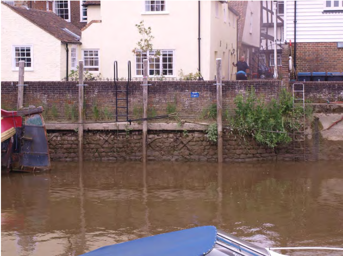
Plate 1: Section 1 of the river wall showing stone walling to the rear of Dolphin Quay
