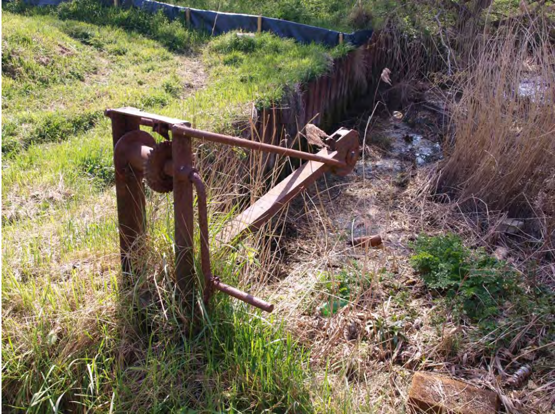
Plate 15: Winch mechanism for sluice
