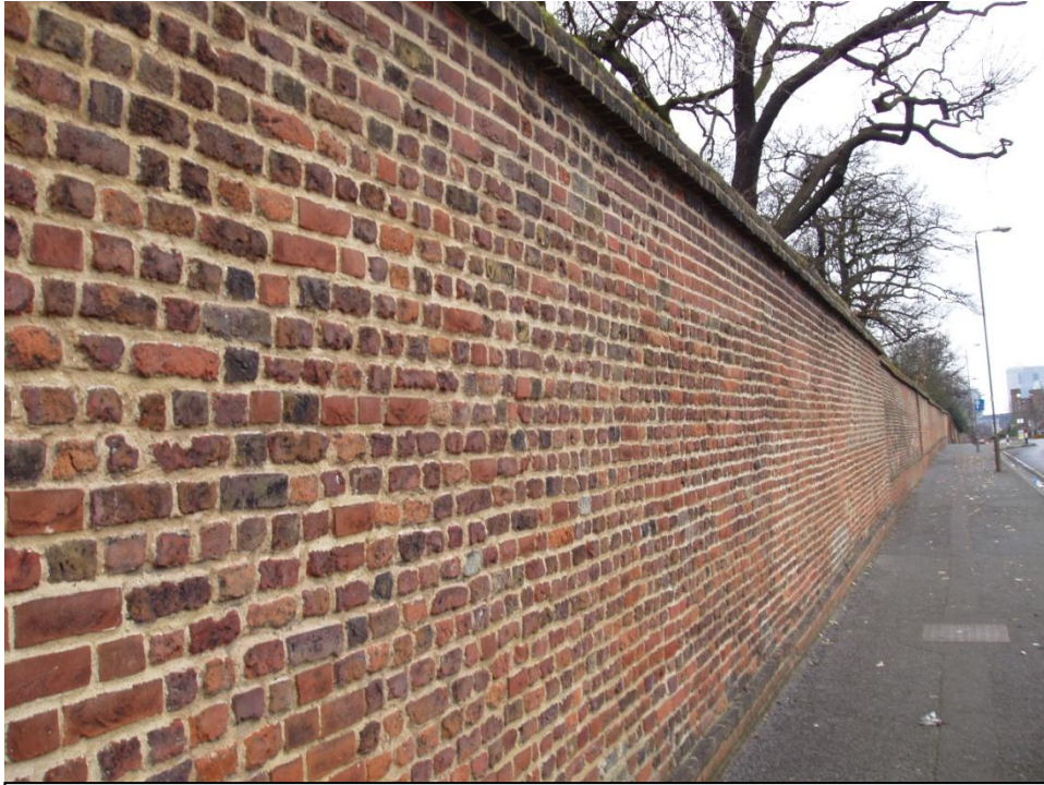
(a) Greenwich(39) park wall. towards the south east corner, this stretch faces east overlooking Blackheath. It is unclear how much of the wall is original because of repairs and repointing since it was built c.1614 23 February 2009
