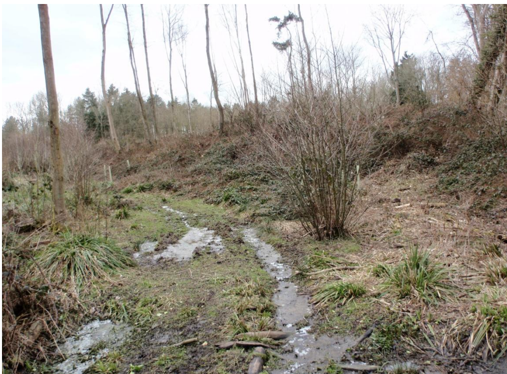
(b) The front of the dam which once held back water for a series of five interlinking fishponds at Halden(41) park. This dam and the whole system were extensively repaired in 1571. 8 March 2010
