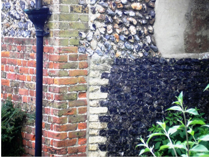
The variety of materials in the walls of The Cottage (originally 1 & 2 Upton Cottages).
