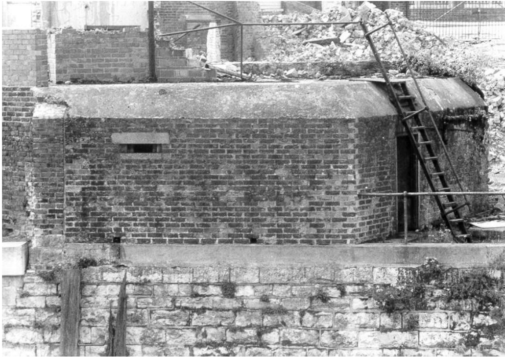
Pillbox at the Style & Winch Brewery in St Peter's Street photographed during its demolition in 1997 (ADS Defence of Britain Database)
