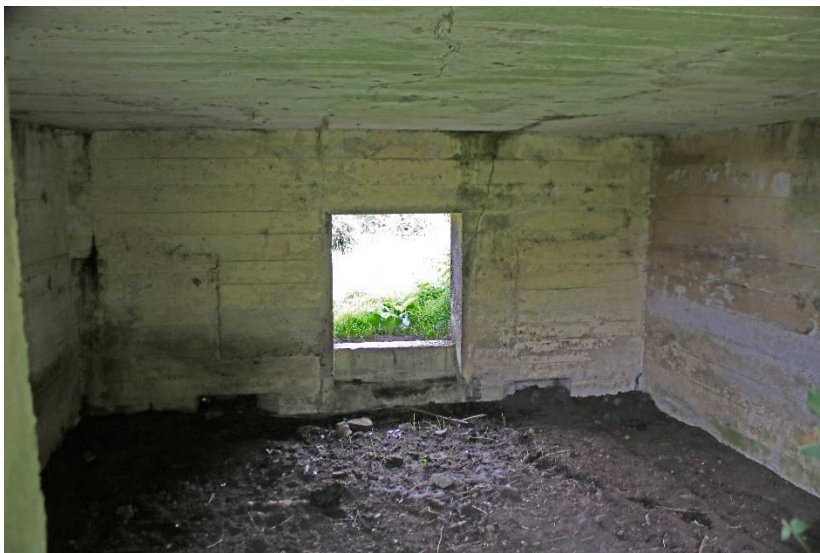
Internal view of the Type FW3/28A at Teston showing the A/T gun embrasure
