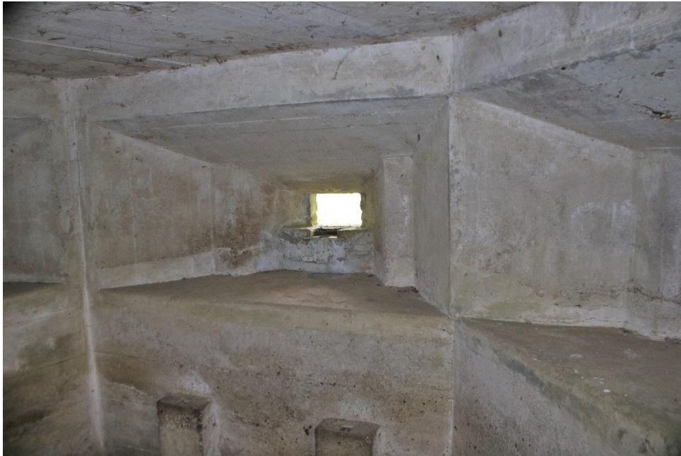
Internal view of one of the embrasures of the FW3/24 at Teston. Note the supports for a Bren gun bipod
