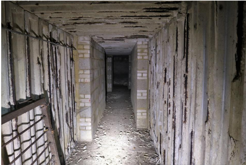
Internal view of the MGS shelter
