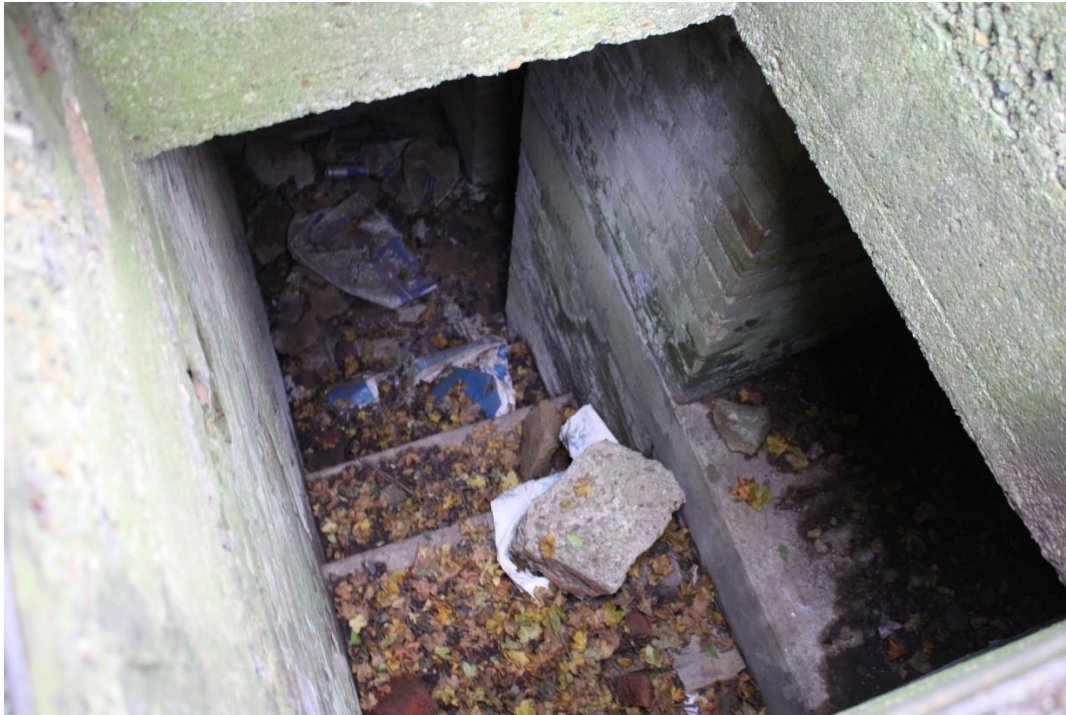
Detling B.H.Q. view into the escape hatch showing the steps up to the Observation Room
