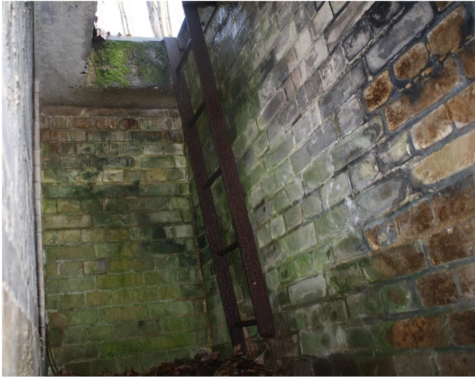
Emergency escape hatch
