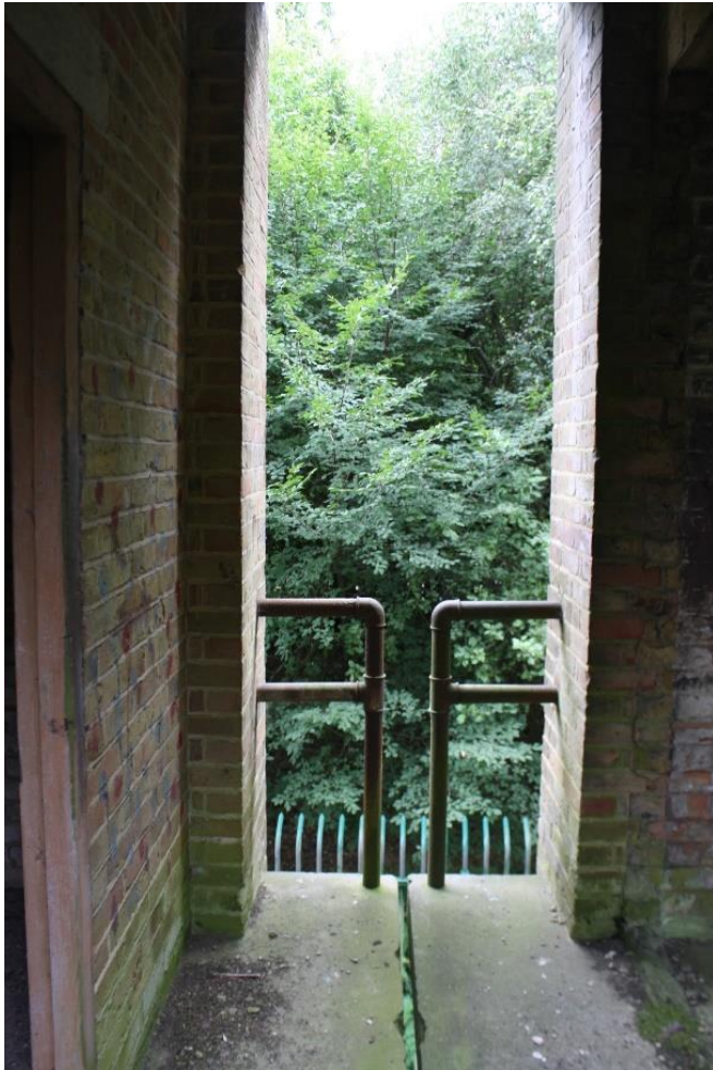
Landing connecting the two towers. Note the gap between the cantilevered floors.
